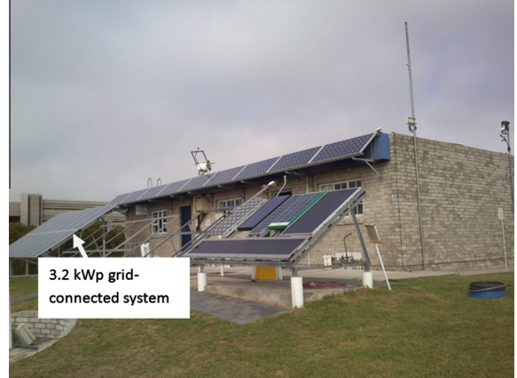
Fig. 1. View of the 3.2 kWp grid-connected PV system installed at the Outdoor Research Facility at NMMU.
